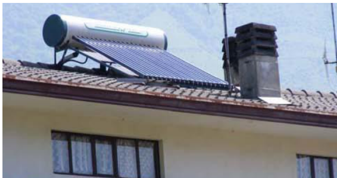
installation on inclined roof
